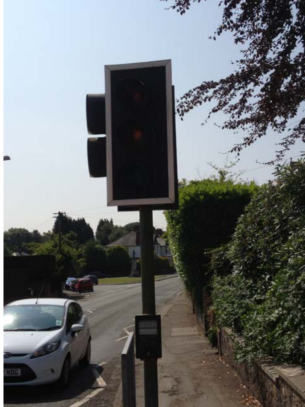
Example of Telematics Defect – (Traffic Signals not working)
