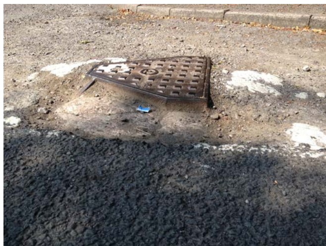
Example of Deterioration Around Ironwork
