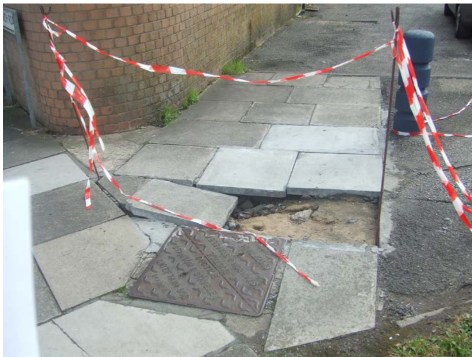
Example of Paving Defect
