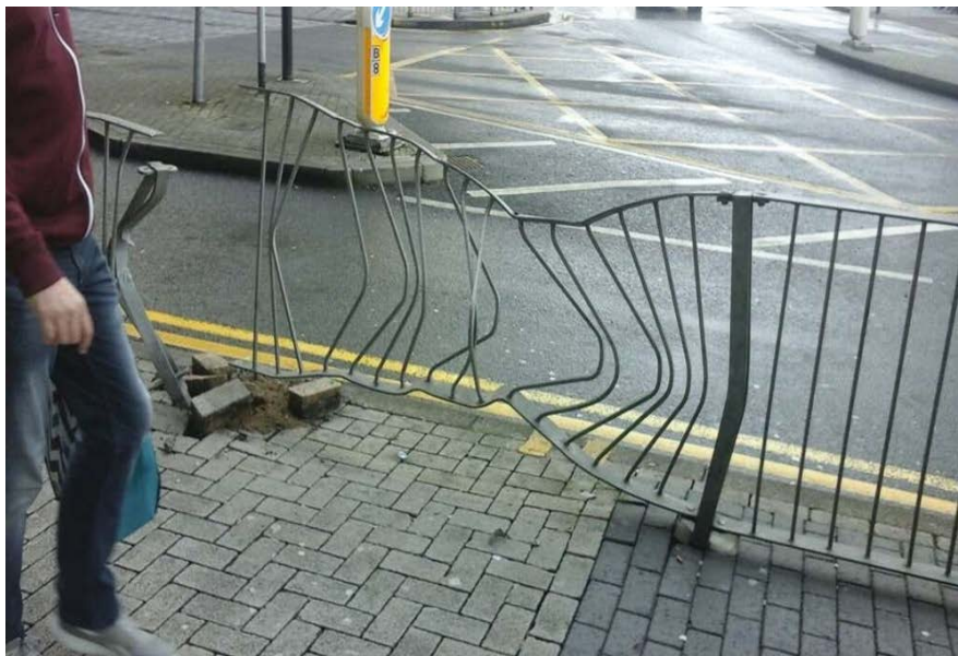
Damaged Pedestrian Barrier
