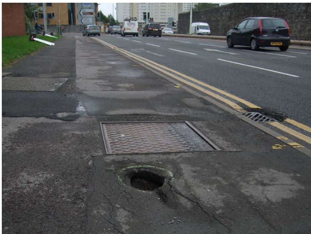
Example of Void
