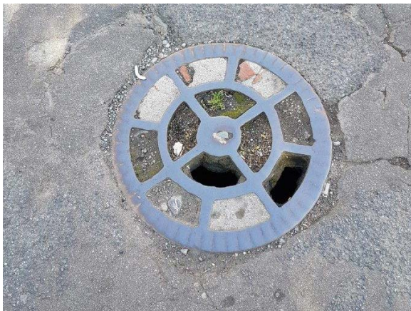
Ventilated drain cover
