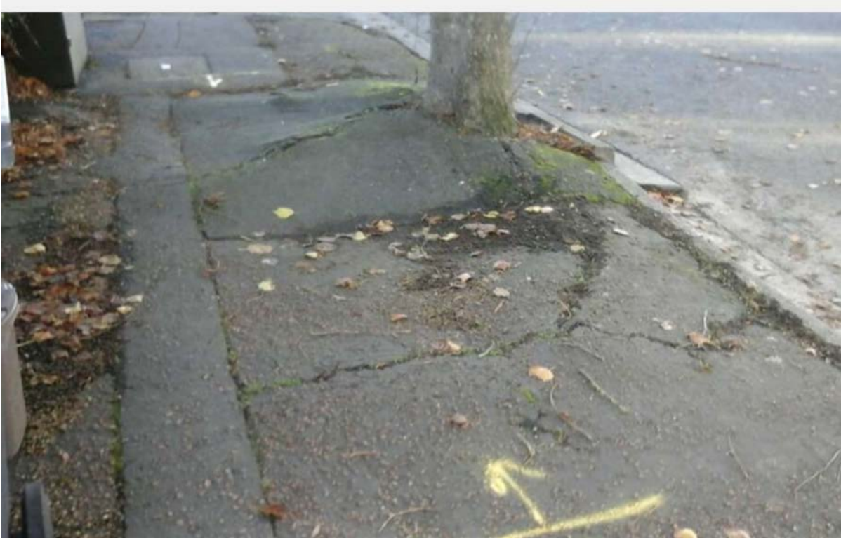
Example of Tree Root Damage
