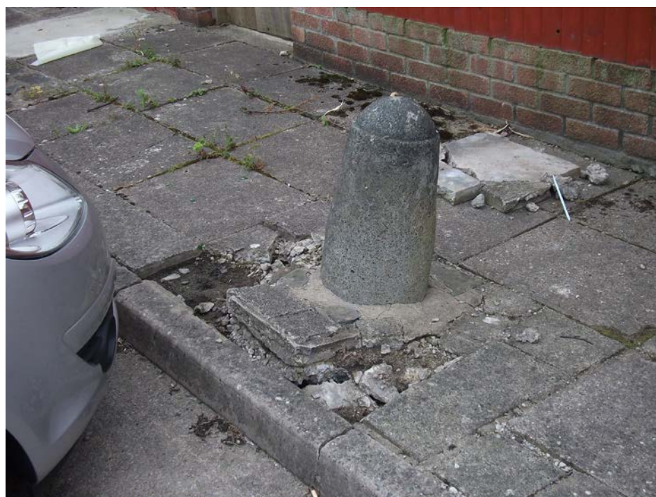
Example of Paving Defect
