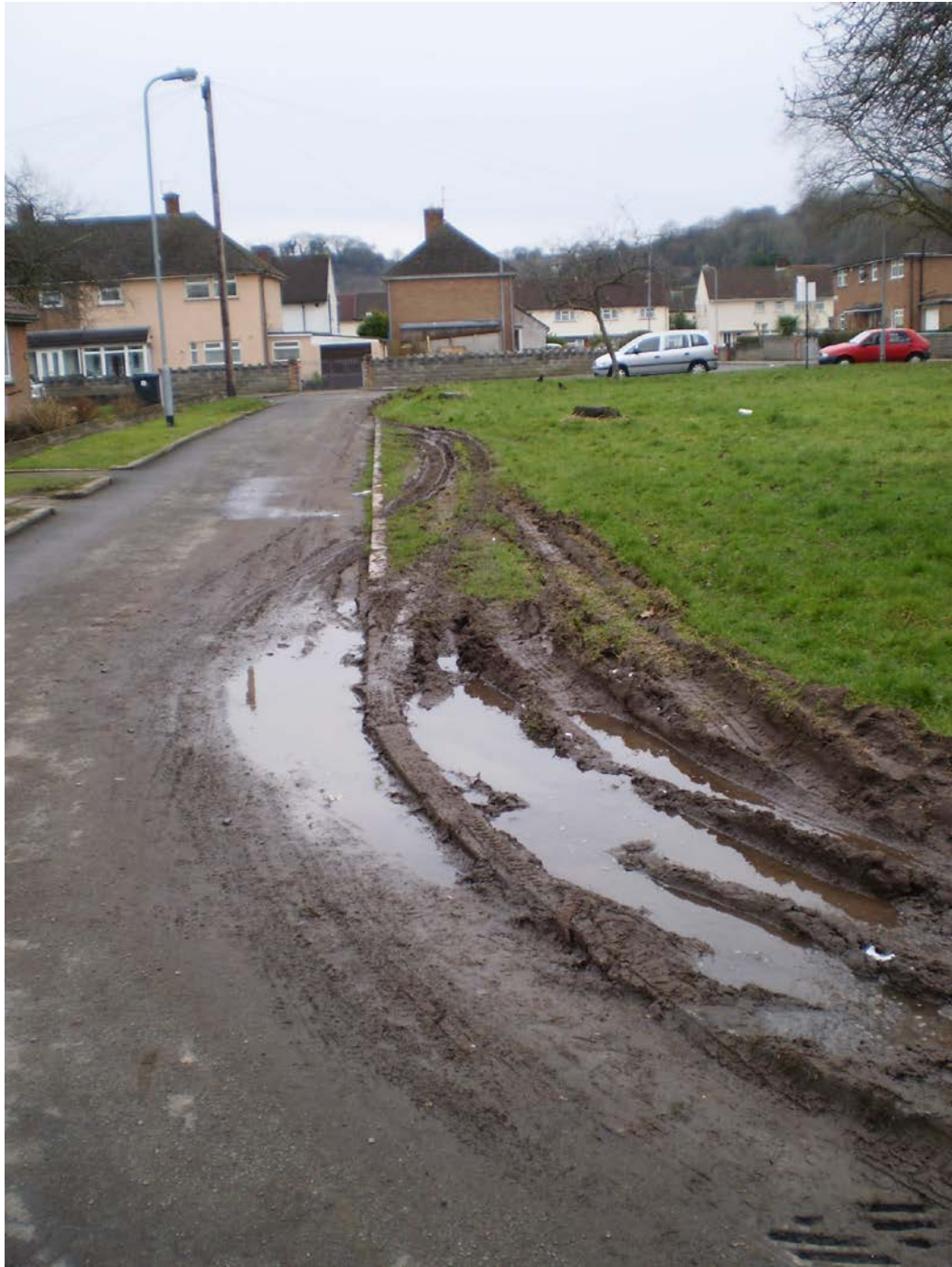
Example of Verge Defect
