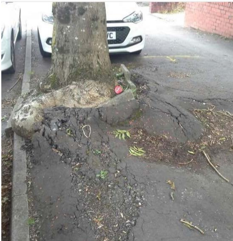
Example of Tree Root Damage
