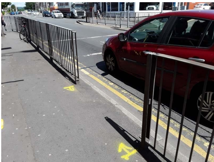
Missing Pedestrian Barrier
