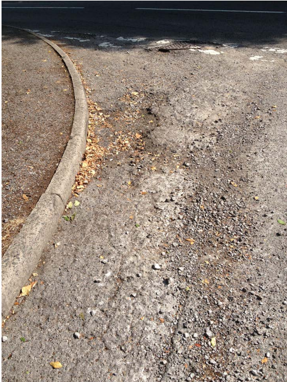
Example of Localised Surfacing Deterioration
